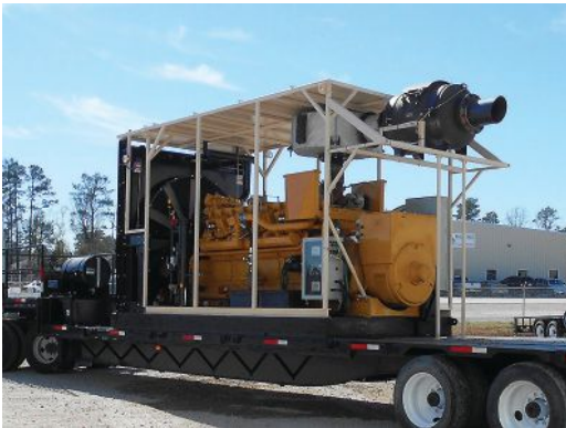
Some of the integrated power systems provided by Global Power Supply
